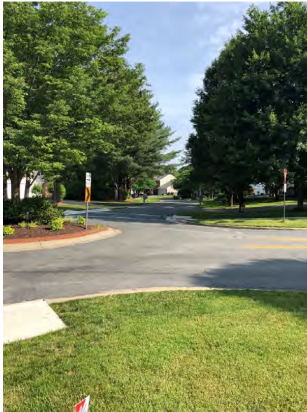
8. Missing crosswalk on east leg of Cherry Valley Dr and Macduff Ave roundabout
